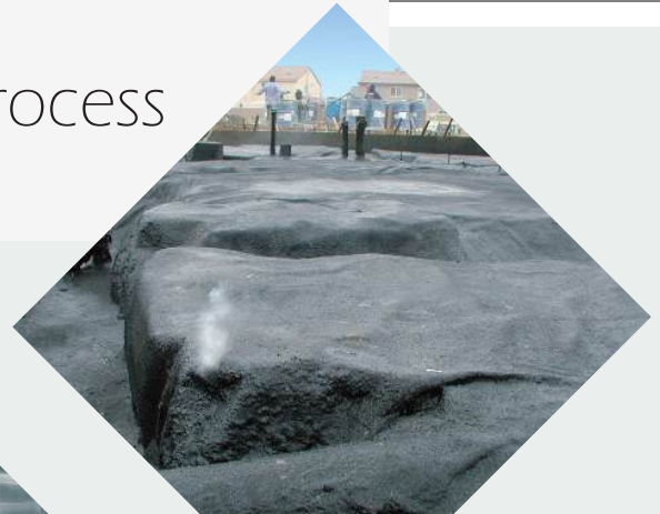
Puncture detected by exiting smoke.
